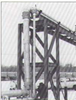
10" Steam and 4" Condensate Series "P2" Ball Joints with Type B Packing Cylinders installed in piping at a trestle over a roadway. Ball Joints are shown with ATS removable Insulation Blanket. 65 - 4" to 12" Ball Joints were furnished to NRG Energy,* Stillwater, MN.
