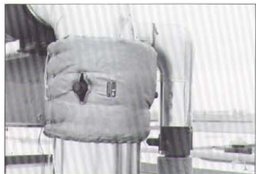
Close-up of 10" Series "P2" Ball Joints with insulation blanket. Note cutouts for access to Type B Packing Cylinders. Blanket for 4" Condensate not yet in place.
