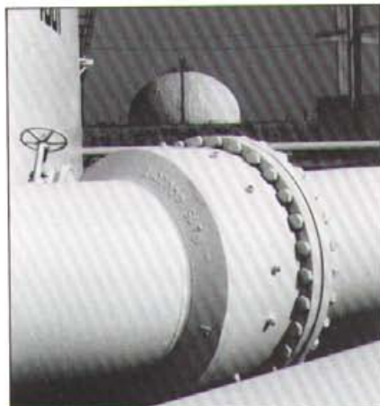
30" Series "S1" Ball Joints installed at AMOCO OIL CO., Texas City Refinery to accommodate tank settling and thermal expansion of a pipeline containing Gas Oil at 150 PSIG/200° F. A total of 32 Ball Joints were furnished, eight each 12", 18", 24" and 30" sizes.
