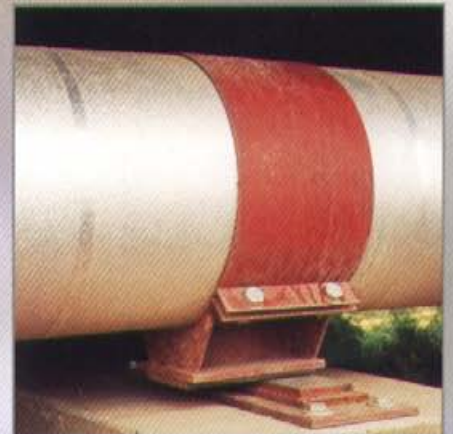
10" Pre-Insulated Pipe Support
